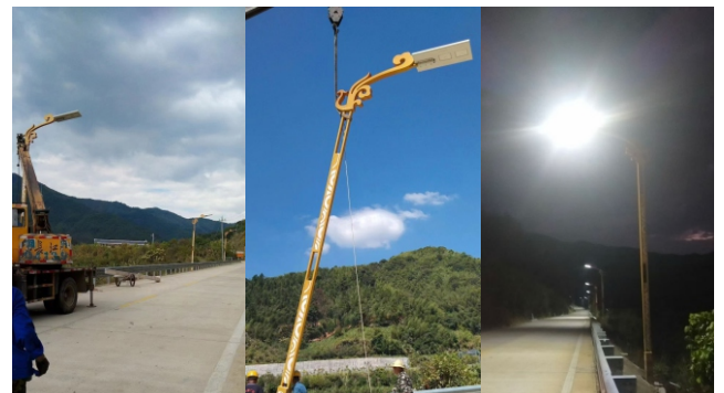
30W Solar Street Light Fu County, Yan'an City, Shaanxi Province, China
