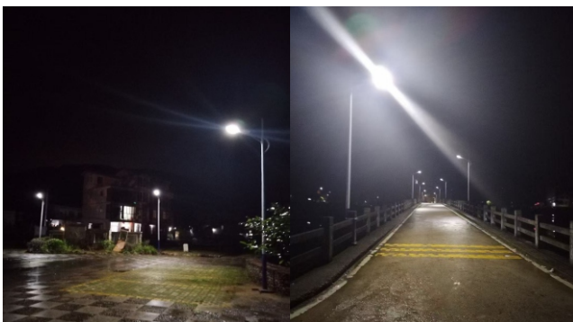
30W Solar Street Light Zigui County, Yichang City, Hunan Province, China
